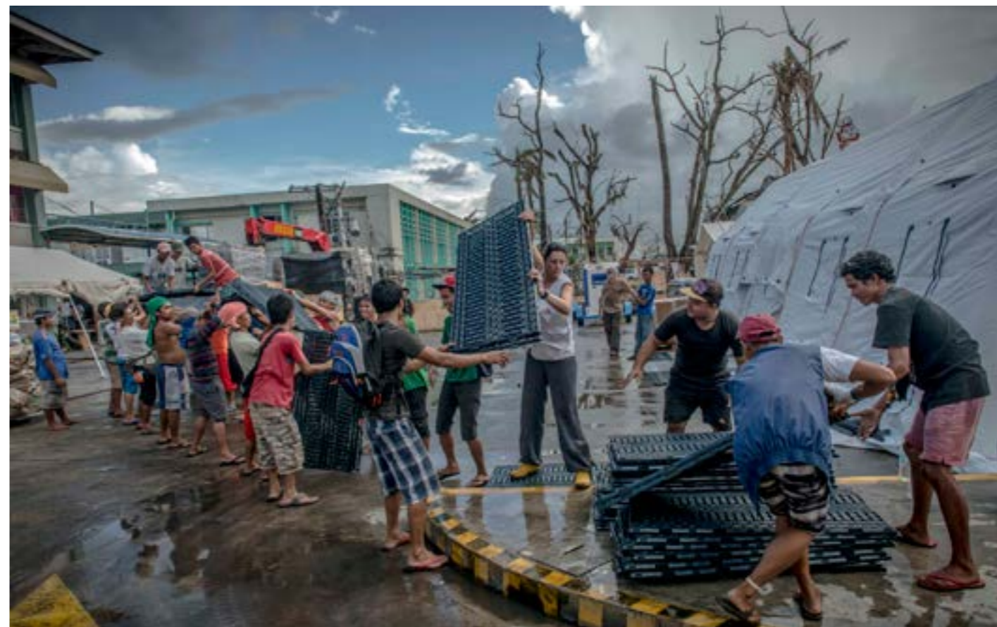
MSF's inflatable hospital under construction, Tacloban. The hospital consists of four inflatable tents with an emergency room, woundcare room, pharmacy and up to 45 hospital beds. Photograph © Yann Libessart/MSF
